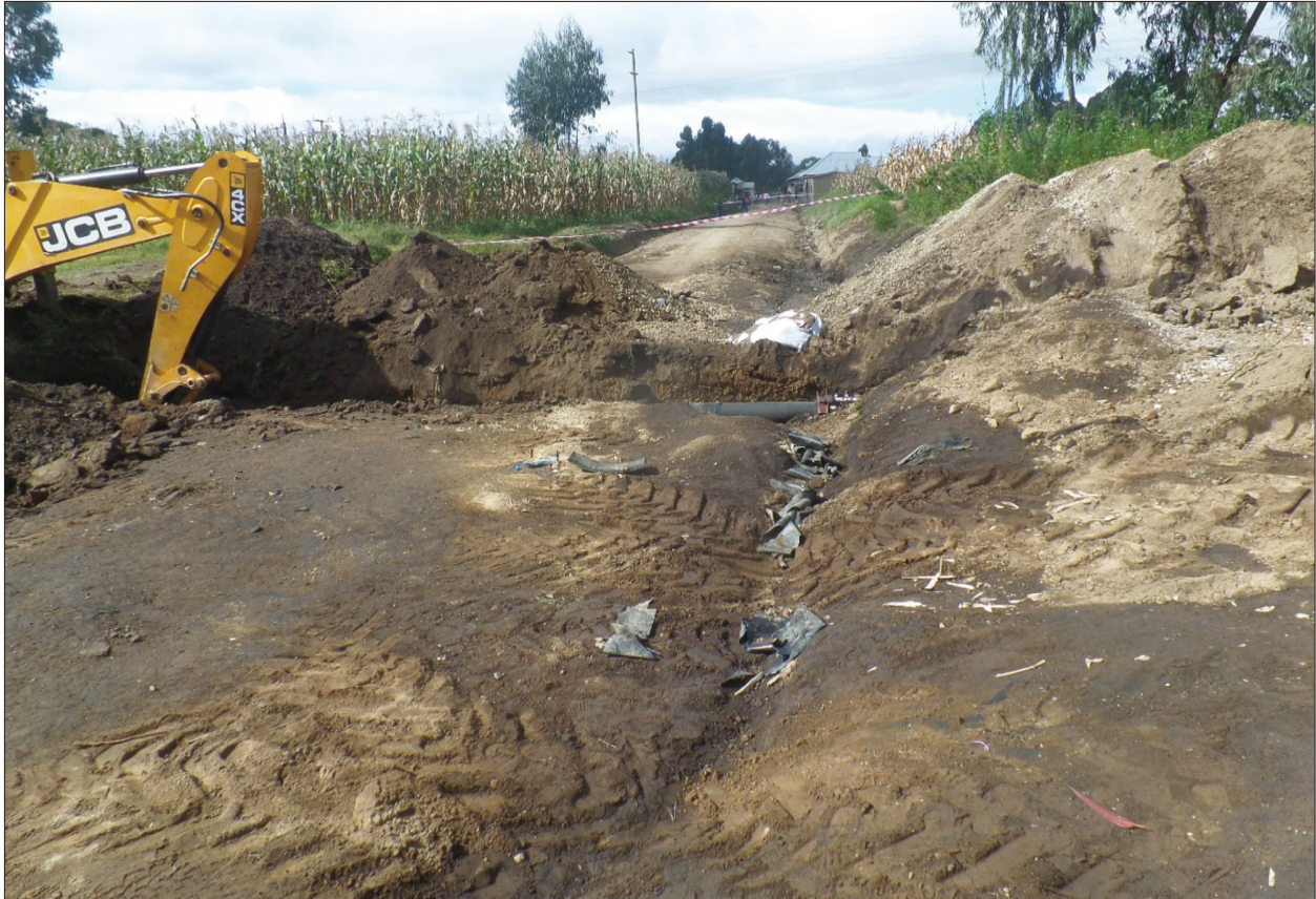
Figure 32: The pipeline's road-crossing where the TARURA contractor was undertaking excavation for the construction of a road and eventually damaged the pipeline. The part of the land was polluted with spilt diesel.
