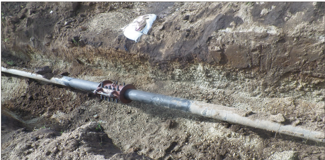
Figure 33: The damaged part of the pipeline was temporarily fixed before connecting the pipeline with the spool piece of the pipe.
