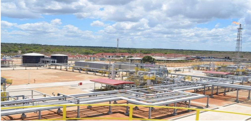
TPDC Madimba Processing Plant with a capacity of 210 mmscfd
